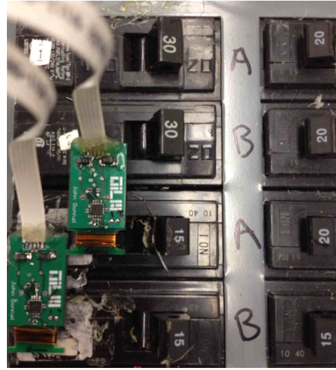
Fig. 13. Monitoring a circuit breaker panel with TMR sensors
