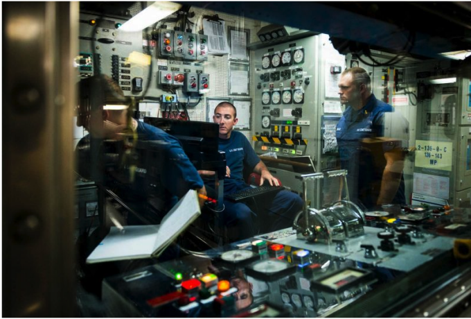
Figure 1. Typical USCG engine room watch. Notice the logbook, termed the "rough log," used to keep machinery operation times and log critical events. Also note the watchstanders monitoring equipment while simultaneously attempting to maintain logs.
