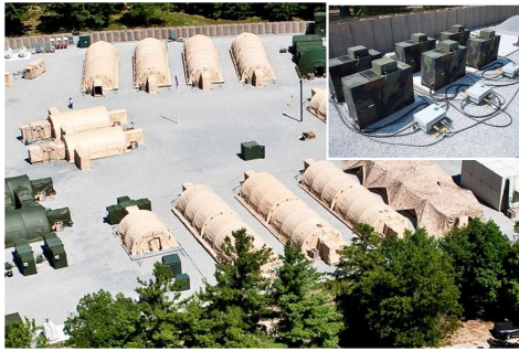
Fig. 1. Aerial photograph of the BCIL; the inset photo in the upper right shows interconnected generators powering the BCIL microgrid.
