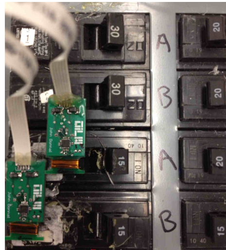
Fig. 15. Monitoring a circuit breaker panel with TMR sensors
