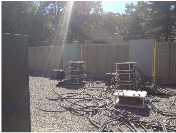
Fig. 2. Ad-hoc power distribution network at Fort Devens, MA
