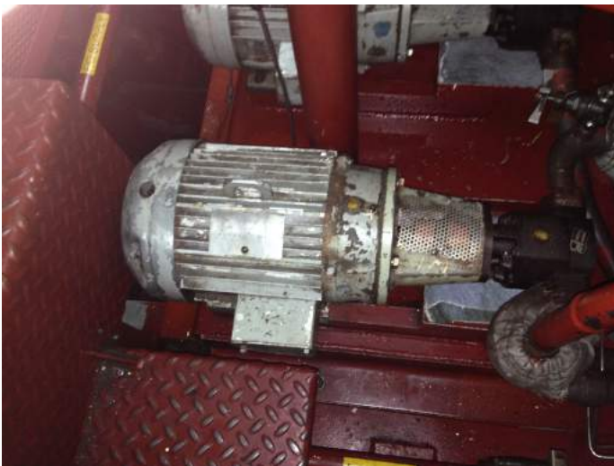
Figure 5. CPP "C" pump motor that supplies pressure to vary the pitch on the blades of the propeller. These pumps are energized when RMD is set and the vessel enters a time of increased risk and fatigue for the crew.
