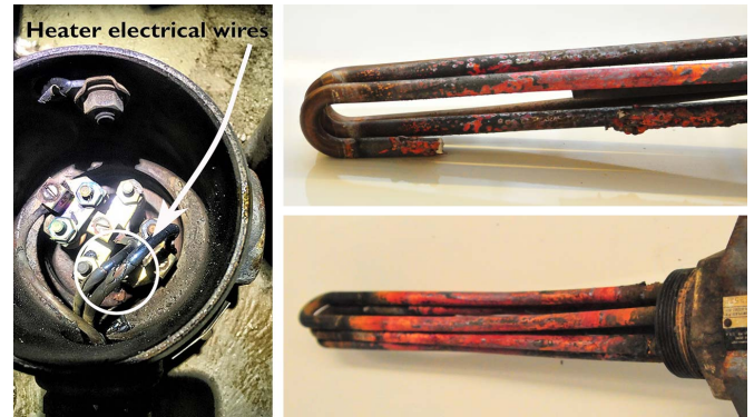
Fig. 15. Left: Bare wiring found in SPENCER port inboard jacket water heater. Right: Jacket water heaters removed from engines after electrical degradation was observed, revealing severe corrosion (top from ESCANABA port inboard heater, removed April 2019, and bottom from SPENCER port inboard heater, removed December 2018).
