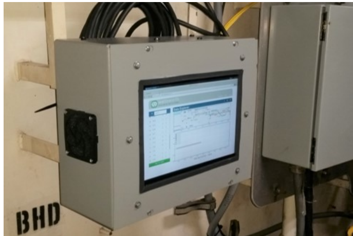
Fig. 2. NILM installation on SPENCER, containing a data acquisition unit and host computer in a single box. Cables connect to the the electrical panel where current and voltage sensors are located.
