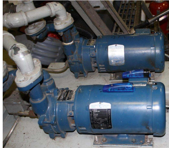
Fig. 10. Two vacuum pumps in the engine room on the ESCANABA . The motor in the foreground will be referred to as Motor A. The motor in the background will be referred to as Motor B.
